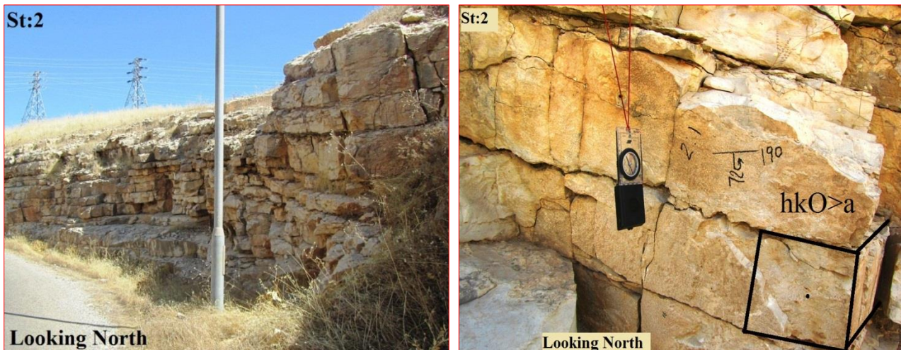
Fig. (13): Two field photos for the joints in the station 2.
