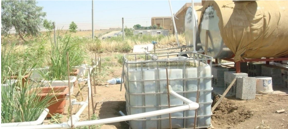
Plate (2): Sedimentation unit
